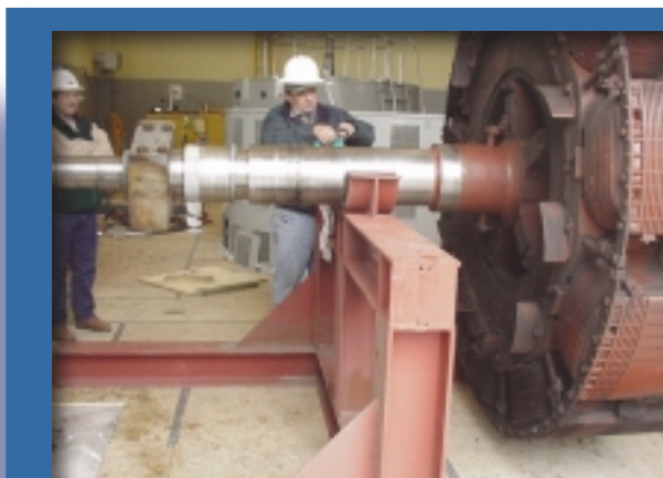
Chugach prepared one of the generator rotors for shipment to General Electric Co. in Utah. The rotors from both of the Cooper Lake Power Plant units were rewound, returned to the plant and re-installed.
