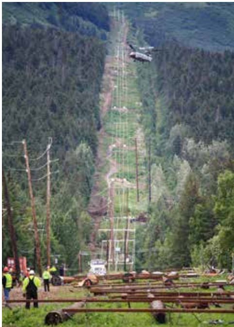
Chugach rebuilt a six-mile section of transmission line between Powerline Pass and Indian.
