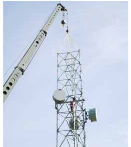
Chugach raised the height of its communications tower at the University Substation to provide a microwave link for the future Hane Substation being constructed on the Anchorage Hillside.
