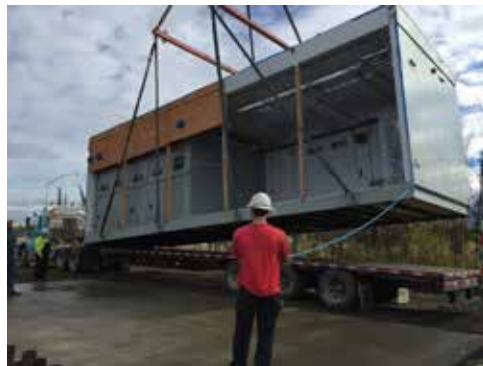
New metalclad switchgear was installed as part of the rebuild of the Dowling Substation.
