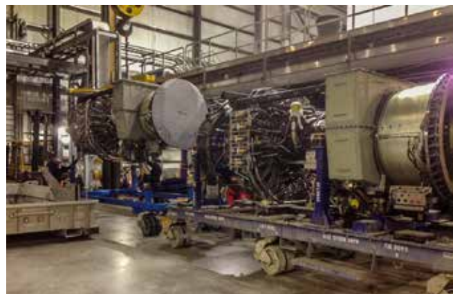
In November a Chugach crew, with the assistance of an on-site GE representative, performed the first engine swap at the Southcentral Power Project. Swapping engines is a planned activity that occurs after so many hours of operation and allows the plant to continue full production while crews perform maintenance offline on the turbine.
