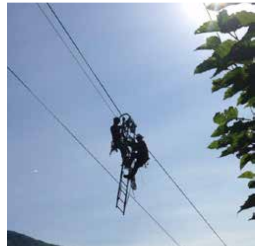
Chugach linemen installed a sleeve to repair broken strands of conductor on one of the phases of the 115-kv transmission line along the Seward Highway.
