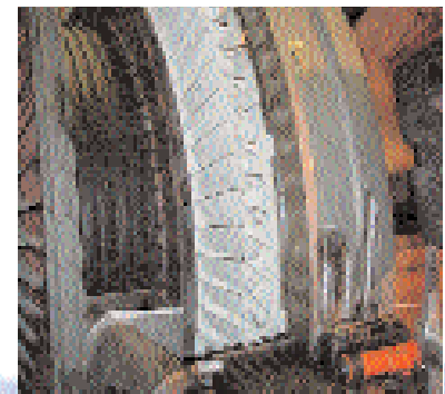
Chugach replaced components on the first-stage nozzle on Beluga Unit No. 5 as part of a major maintenance project.
