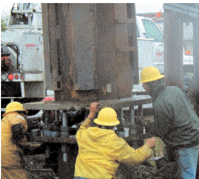
Chugach relocated major electric lines along Dowling Road between the Old Seward Highway and Lake Otis Boulevard in conjunction with a State of Alaska construction project. Road construction is scheduled to start in the spring of 2003.
