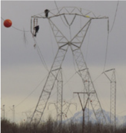
A transmission tower near Dynamite Slough on the Susitna River was moved to prevent damage from erosion.
