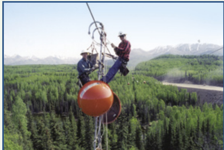
Chugach linemen replacing a lighted aircraft warning ball on a 230-kilovolt transmission line.
