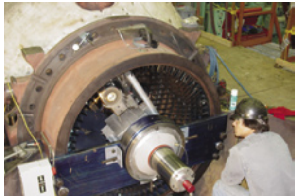
A Beluga Power Plant employee aligned the newly-installed rotor during the Unit 6 Overhaul.
