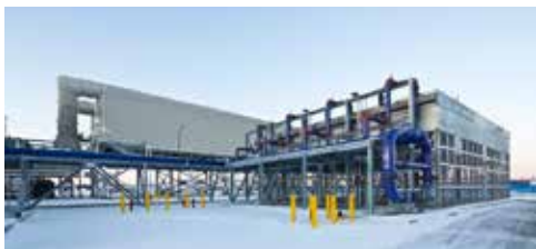
Rate adjustments to recover costs associated with the Southcentral Power Project and benefits from its fuel efficiency were put in place in 2013.
