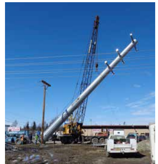
A portion of a 138-kv transmission line was relocated to make room for an upgrade of Dowling Road between the Old Seward Highway and C Street.
