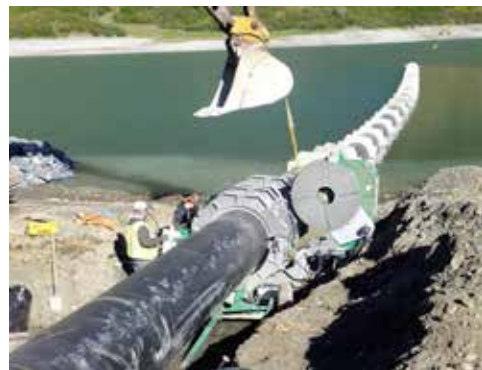
A diversion structure and two miles of buried 36-inch diameter polyethylene pipeline were installed in 2013 to carry water from Stetson Creek into the Cooper Lake reservoir. Infrastructure to allow the release of warmer water from the reservoir into Cooper Creek will be constructed in 2014.
