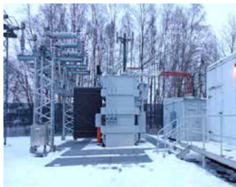
A new substation transformer was installed at the Turnagain Substation to replace one nearing the end of its useful life.
