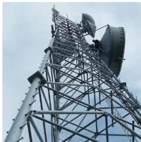
Chugach continued a multi-year project to replace its microwave radios with new units with enhanced communications capabilities.
