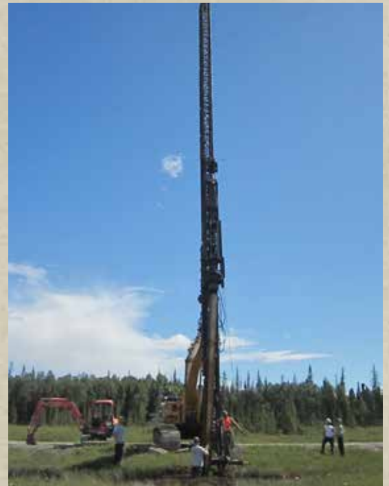
One of the largest line extension projects in recent years took place in the fall at Tyonek, where about a mile of both 3-phase and single-phase distribution line was added to the system to support ongoing economic development activity.
