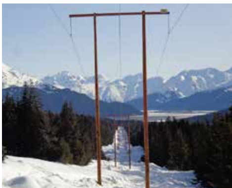
A $15 million grant from the Legislature, administered by the Alaska Energy Authority, paid for a Chugach project that rebuilt 15 miles of transmission line up and through Ternagain Pass.
