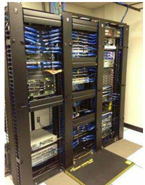
The new core switch installed and configured by Information Services is the heart of Chugach's computing network.
