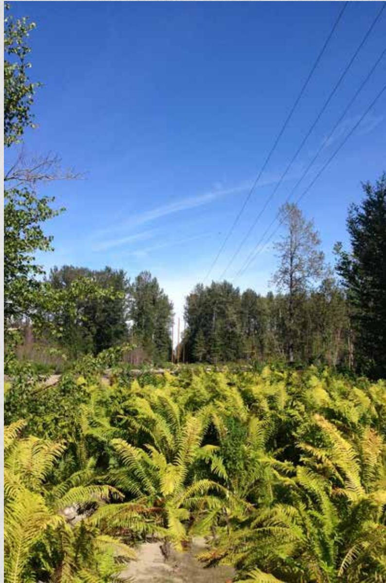
Front cover: Chugach crews installed aerial marker balls on a newly constructed section of distribution line over the Chuitna River. Above: The new line replaced a temporary crossing erected after flooding in September 2012 damaged the line.
